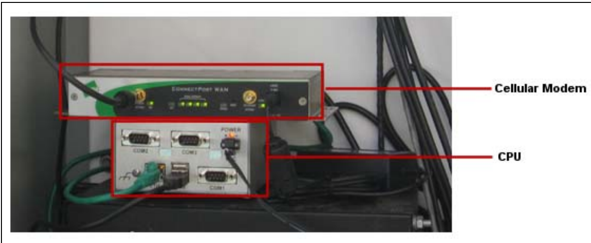
Figure 16. South Main Cabinet Deployment
